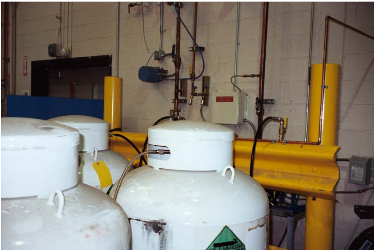
Figure 4: C_3F_8 cylinders connected to gas distribution system
